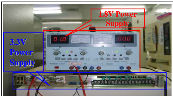
External Power Supply
